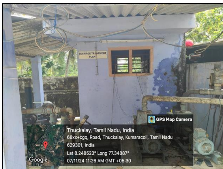
Sewage treatment plant were observed in the campus
