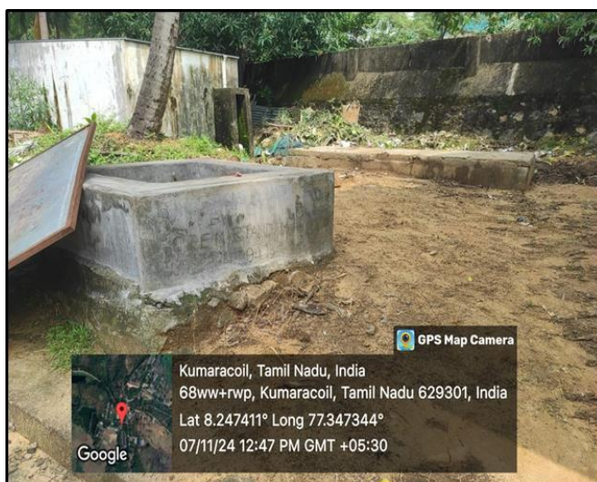
Biogas plant observed in the campus
