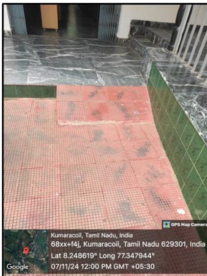
Ramp walk facility observed for the comfort of person with disability.
