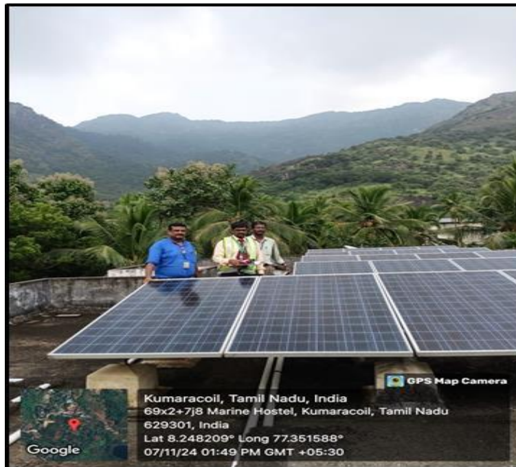
Solar panel observed in the campus
